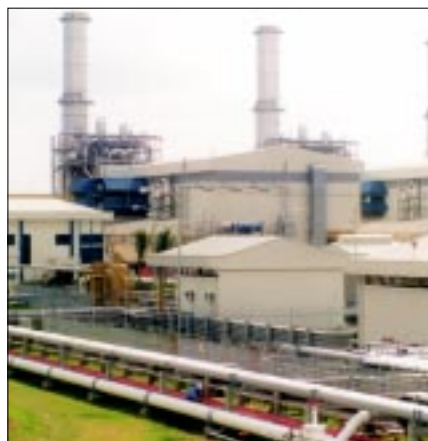
Figure 3: Units 1 and 2 of the first Block were simultaneously commissioned on diesel oil in mid February
