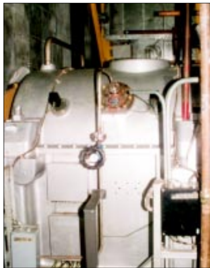
Figure 6. Without an SSS clutch in each unit simultaneous commissioning would not have been possible
