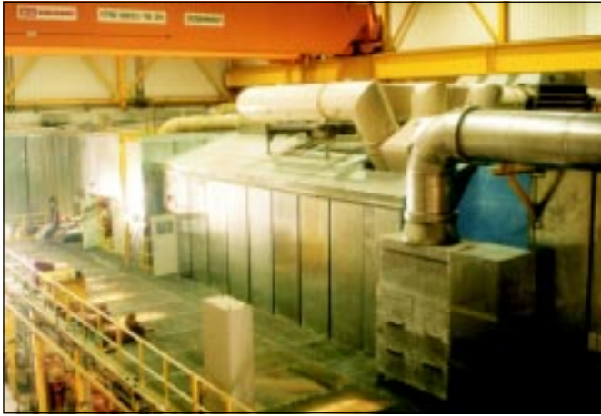
Figure 4: Siemens standard single shaft combined cycle has centrally mounted generator and steam turbine exhausting to axial condenser as can be seen here in left background.
