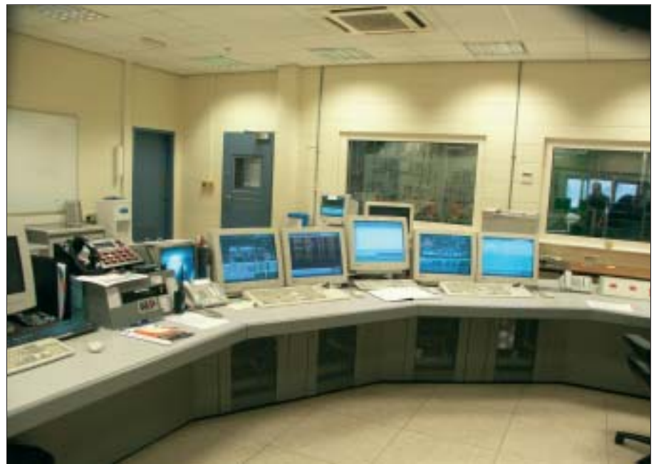
Fig.3 Control room with equipment supplied by by ABB Power Automation is located alongside the turbine hall, visible through windows, and is operated by a 3-man shift crew with supervisor and two control engineers .
