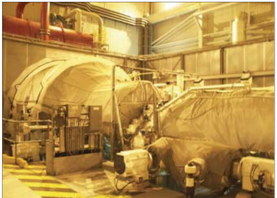
Fig.6 The steam turbine is a 2-cylinder design with combined IP and single flow LP cylinder , which is mounted in a n acoustically lined enclosure. The unit exhausts to a 25-cell air condenser.
