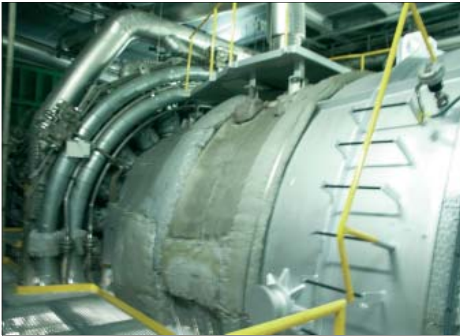
Fig.4 The GT26 viewed from the exhaust end showing the fuel manifolds for the SEV burners. On November 12, when this picture was taken, the gas turbine had been shut down 12 hours and was cooling in readiness for the C-inspection
