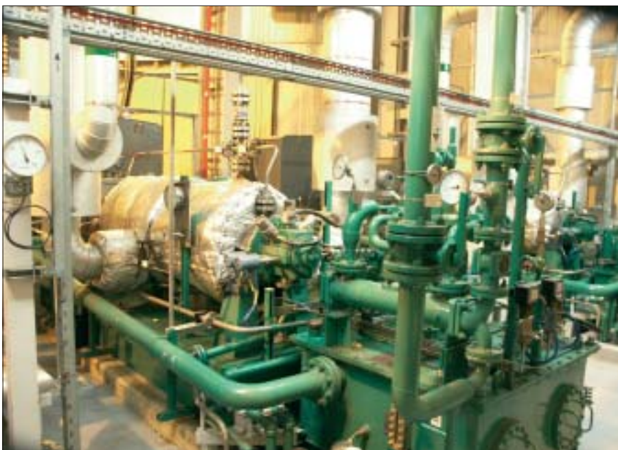
Fig.5 In this power plant, to guarantee high availability 100% redundancy is carried on all pumps. Here can be seen the IP boiler feed pumps supplied by Flowserve from the former Byron Jackson nuclear power factor at Etten Leur, Netherlands.
