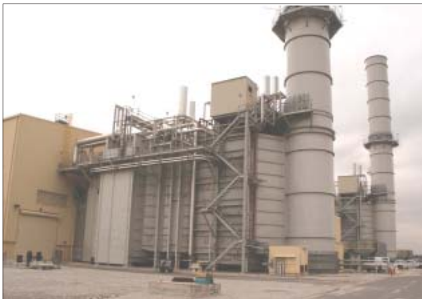
Fig 4. General view of an HRSG showing sound insulation on the once through section. The yellow hut beside the nearer stack is the emission monitoring position which collects data from both stacks to see that NOx is less than 2 ppm
