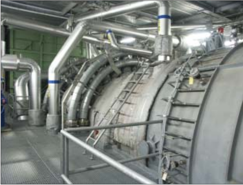
Fig 3. The gas turbine is housed in a spacious acoustic enclosure shown here looking towards the HRSG with the fuels manifold of the first combustor stage at centre and the cooling air bleed pipes leading off to the OTC units.
