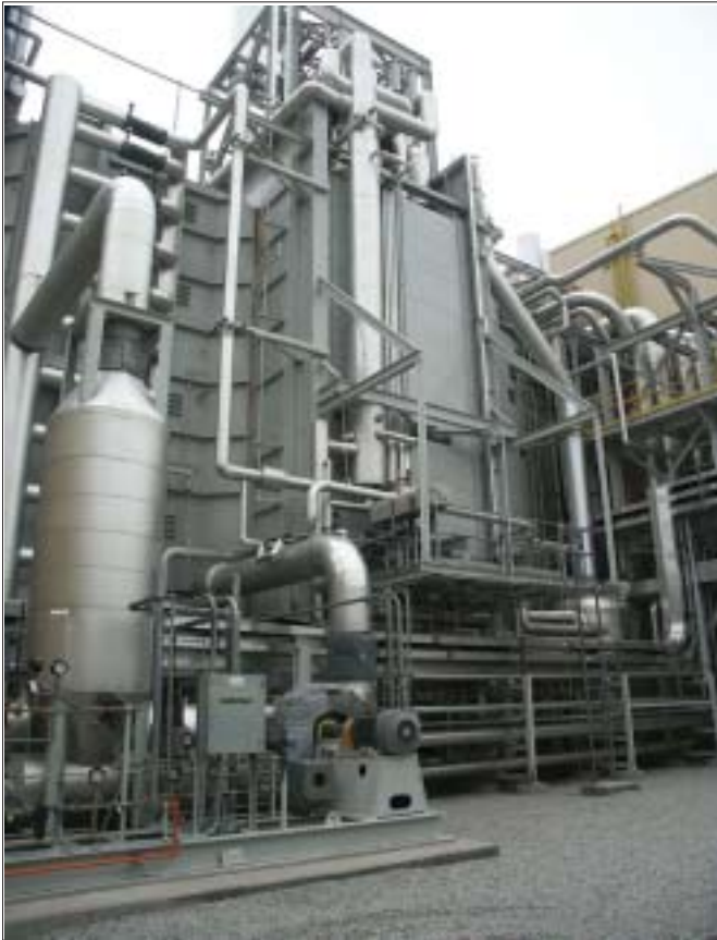
Fig.1 This view of the HRSG shows the once through section , with heavy sound insulation. The long tube in the centre of the picture is the pressurizer with the blow down tank at left.
