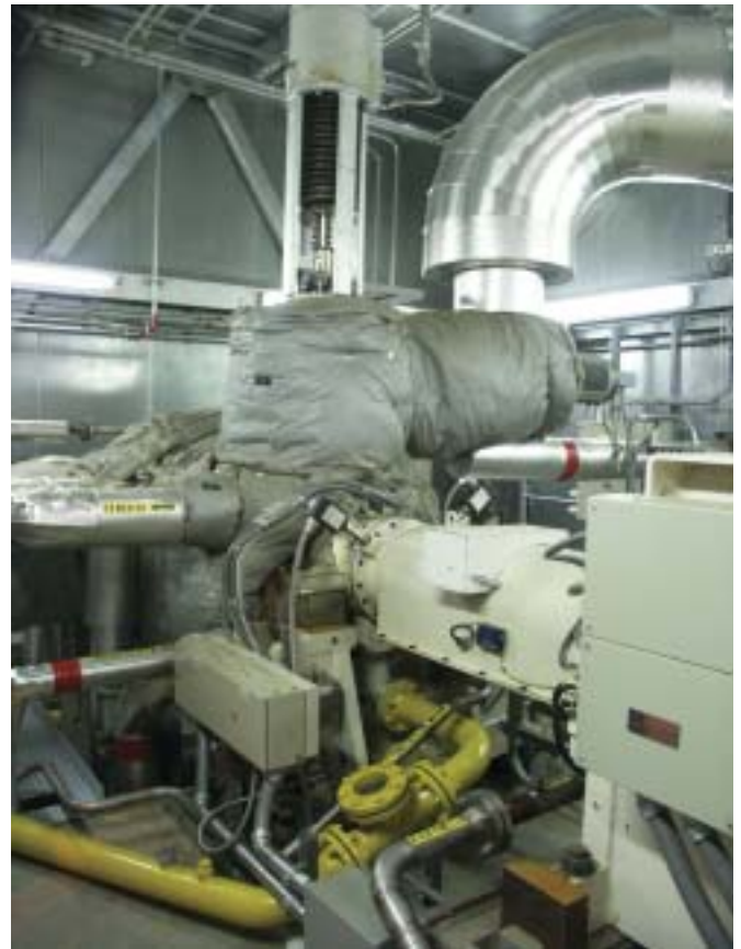
Fig.2. The steam turbine HP in its acoustic housing with the 160 bar steam entering from the left. The gearbox, which drops the speed from 8900 to 3600 rev/min, is at right.
